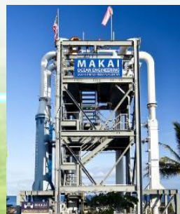
2015 : 100kW OTEC plant Grid-connected (NELHA/MOE)
