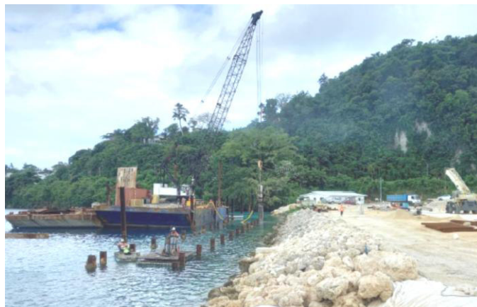
Figure 2 - Additional Ocean Logistics barge and crane in process of the old piles' extraction.
