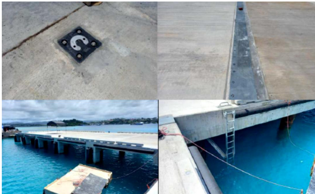
Figure 4: (Top left) Flush bollard on ramp. (Top Right) Seismic separation joint cover plate. (Bottom Left) Fenders, bollards and edge kerbs installed. (Bottom Right) Ladder.
