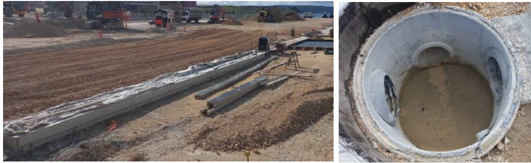
Figure 5 - Left picture shows last section of ACO drain is now complete. Right picture shows earthquake damaged manhole.
