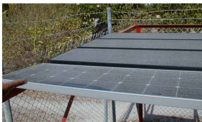
Figure 4-1 - Marakei telecom installation (note the surface dirt)
