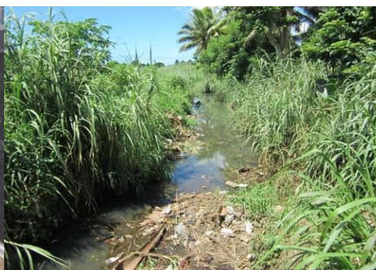
Photo: Balgovinda main drain in Nasinu is choked with debris, silt and vegetation due to lack of maintenance access, causing upstream flooding. A 3km long gravel maintenance access road is needed alongside the drain.
