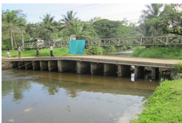
Photo: Quaia Road Bridge on the Lami River has insufficient waterway area. It obstructs flood flows and causes frequent flooding of adjacent upstream Quaia Settlement. The bridge needs to be demolished and raised to reduce flooding.
