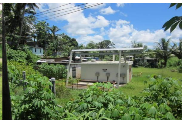
Photo: 10 houses in River Road Settlement near the WAF sewage pump station. When Wainibuku Creek floods, houses are inundated with floodwater mixed with raw sewage from the pump station. Another 56 houses are also flooded. The creek needs to be dredged and the 10 houses relocated.
