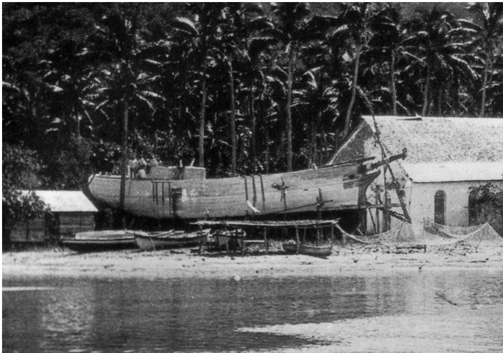
The trading schooner "Takitumu" under construction at Ngatangia in the early 1890s.
